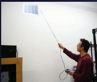
HVAC testing and balancing
